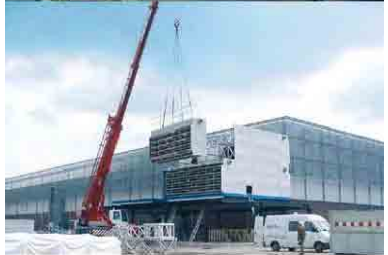
Cross flow cooling tower type XM Telephone/Communication center in the Netherlands
